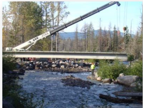
AEC installed a new 315 lineal foot super structure bridge spanning the middle fork of Hood River
