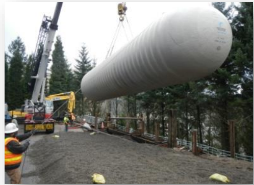
AEC supplied and installed a 30,000 gallon diesel tank at the Veteran's Hospital in Portland, Oregon
