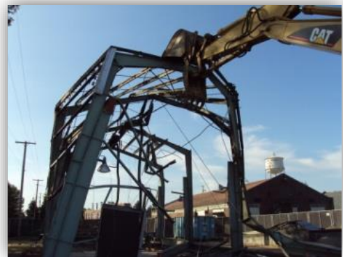
AEC demolished structures and disposed of refuse materials at McChord AFB, including this former locomotive workshop
